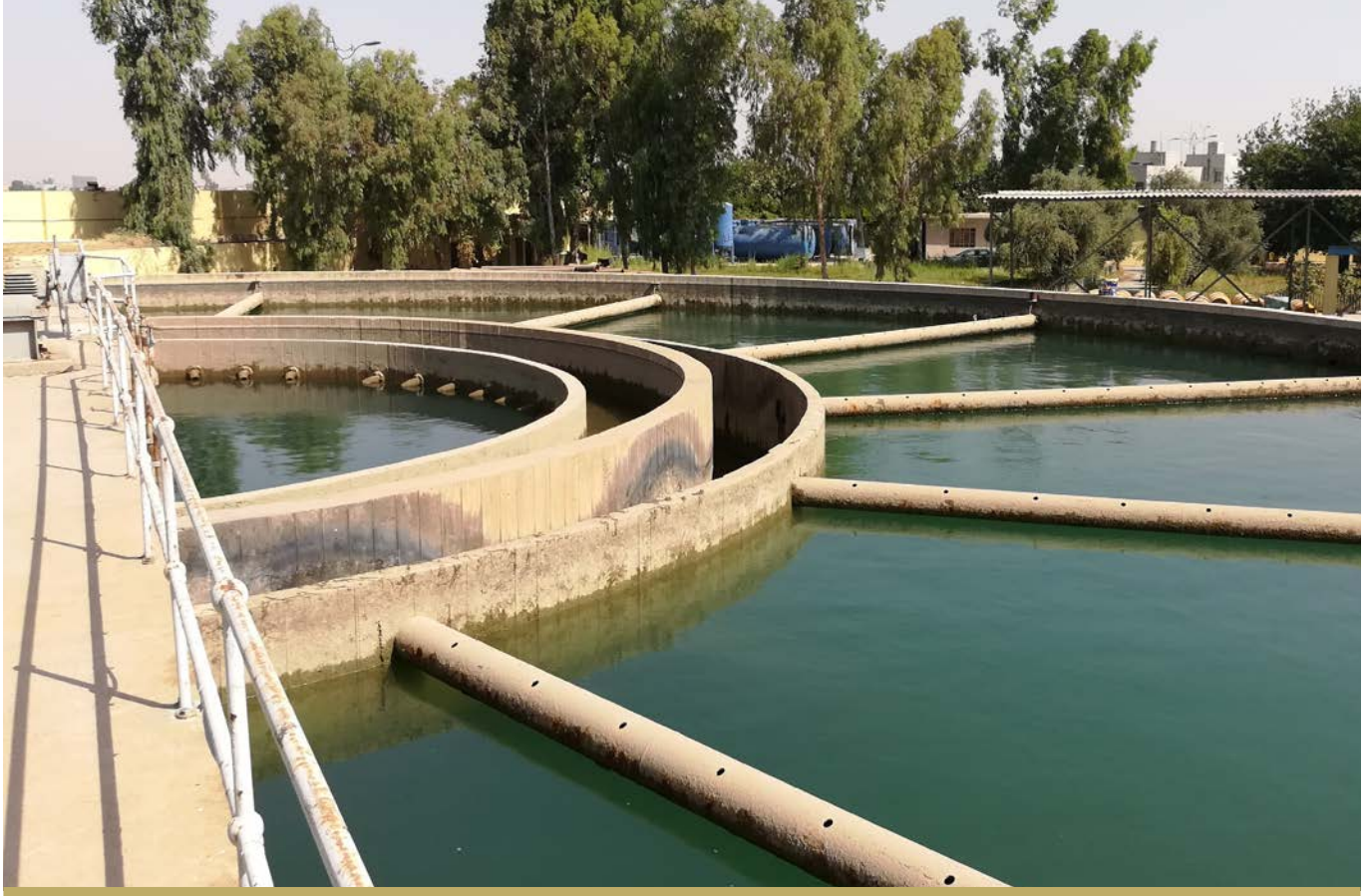
WATER PROVISION IS A CRITICAL PRIORITY IN ALL NEWLY LIBERATED AREAS. REHABILITATION OF THE AL QASOOR WATER TREATMENT PLANT IN EAST MOSUL IMPROVED THE WATER CAPACITY FOR 300,000 EAST MOSULAWIS.
