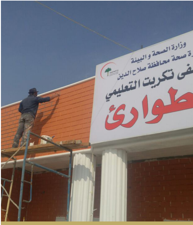
THE TIKRIT TEACHING HOSPITAL IS THE MOST IMPORTANT FFS PROJECT UNDERWAY IN THE CITY.
