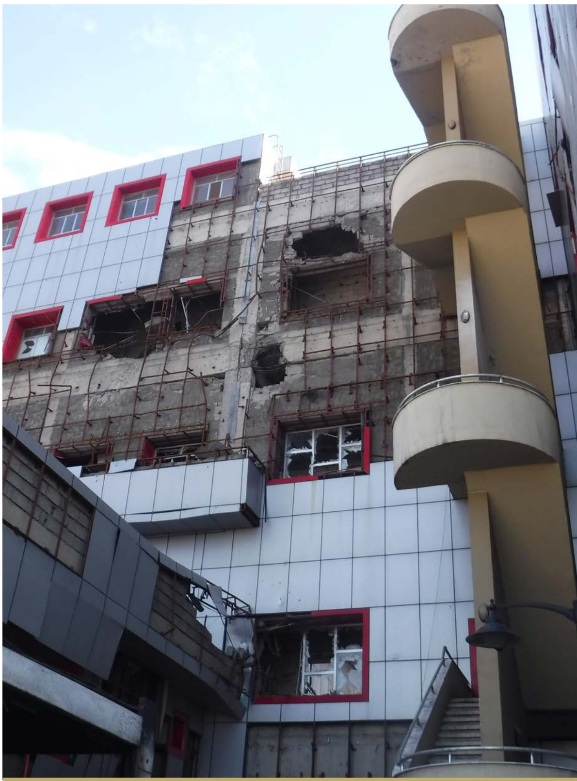
THE QAYARA HOSPITAL WAS SEVERELY DAMAGED DURING THE OCCUPATION OF THE CITY, AND HAD BEEN AN IMPORTANT FACILITY FOR OVER 100,000 NEARBY RESIDENTS. THE FACILITY IS ONE OF THE EXPANDED STABILIZATION PROJECTS OF FFS.
