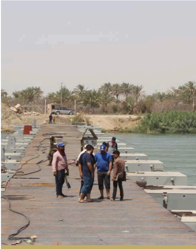
REHABILITATION OF THE AL MA'MOUN FLOATING BRIDGE BY FFS SUPPORTS VEHICLE AND PEDESTRIAN TRAFFIC FOR THOUSANDS OF ANBARIS EVERY DAY.
