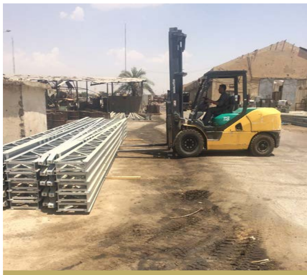
EQUIPMENT SUCH AS POLES AND CABLES HELP THE ELECTRICITY DEPARTMENT OF SHERGAT REPAIR DAMAGED PARTS OF THE NETWORK.
